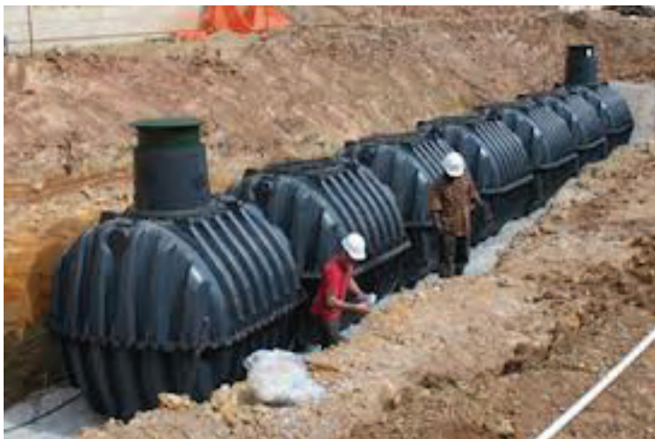
A similar system to the one in the photo was installed at MassMutual.
