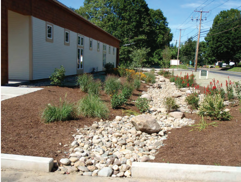
A rain garden along Route 9 in Hadley, captures storm flow from a drive and parking lot. This photo is taken just after installation and before plants are really established.
